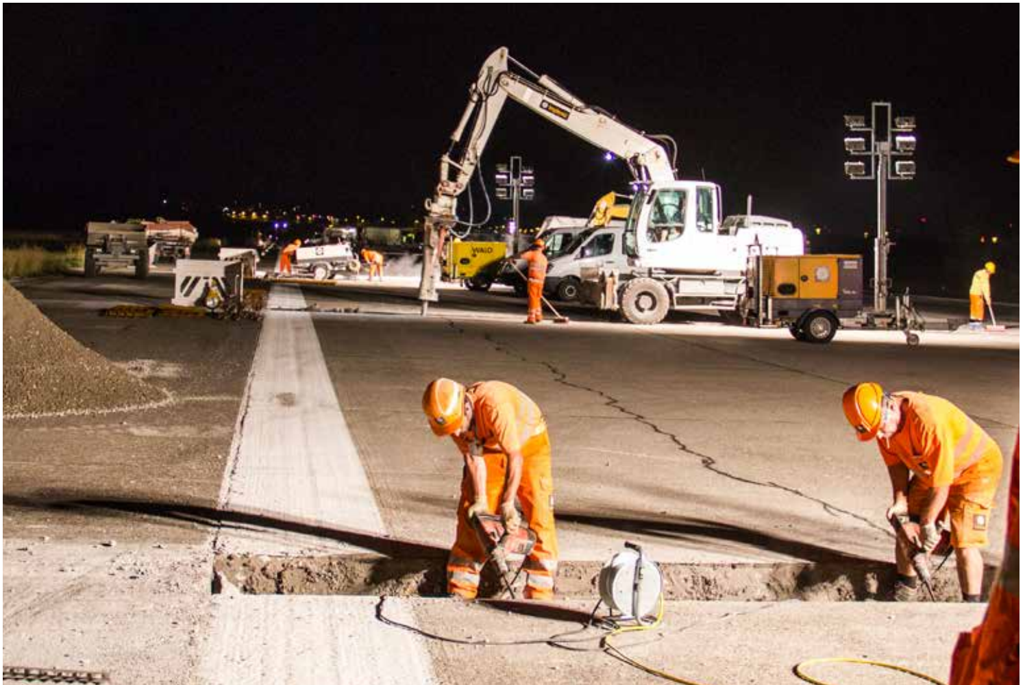
Works are done at multiple trenches at the time. All of them have to be done till 5.30 a.m.
