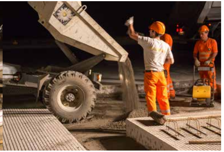
A good sense of proportion comes handy for estimating the lean concrete needed.
