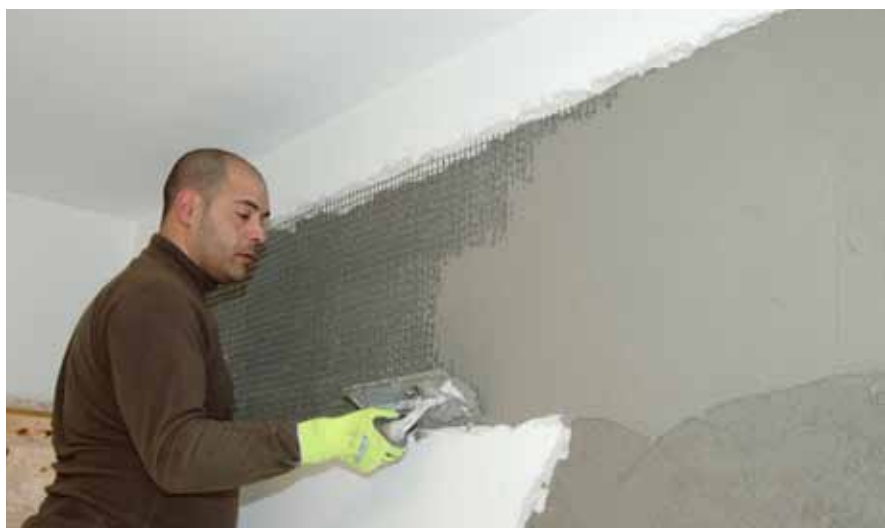
After an earthquake in L'Aquila, Italy: Fixing procedure with Sika® MonoTop®-722 Mur and SikaWrap®-350 G Grid
